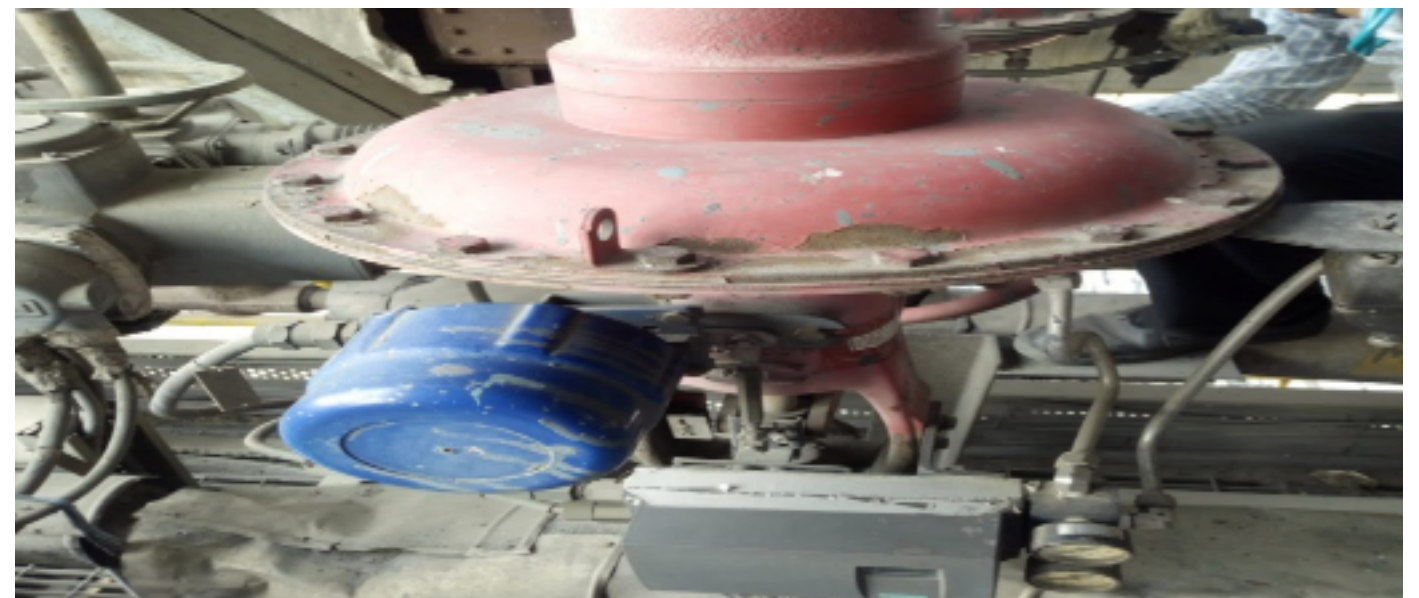
Calibration of Control Valve
